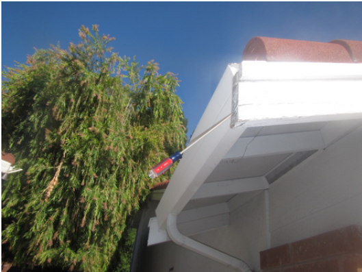
Pest-report photograph: damaged roof-edge wood.
