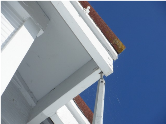
Home-report photograph: fascia / eave deterioration. Coordinate the wood and roof trades.
