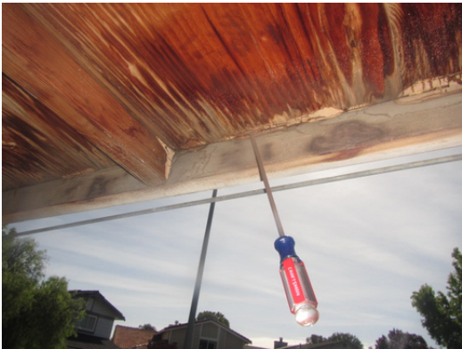
Pest-report photograph: garage-door damage; other trade.
