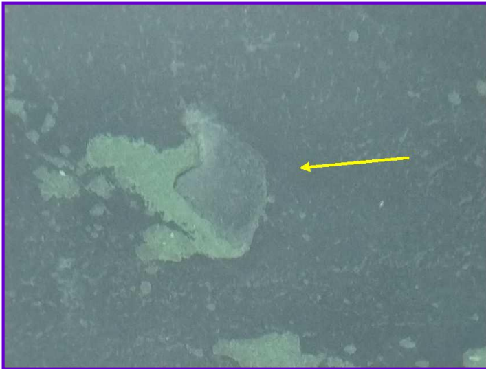
DEFERRED: There are areas of the pool body surfaces that are showing signs of deterioration.
