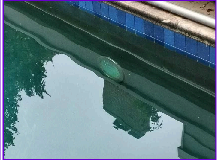
MAINTENANCE: The pool and spa lights did not respond.
