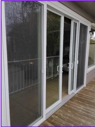
SAFETY: For child safety reasons, alarms are required to be installed at all exterior doors.
