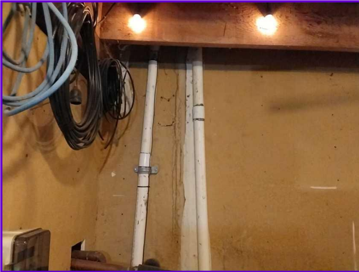
MONITOR: Water stains were observed near the hydronic solar system water line coming from the roof.
