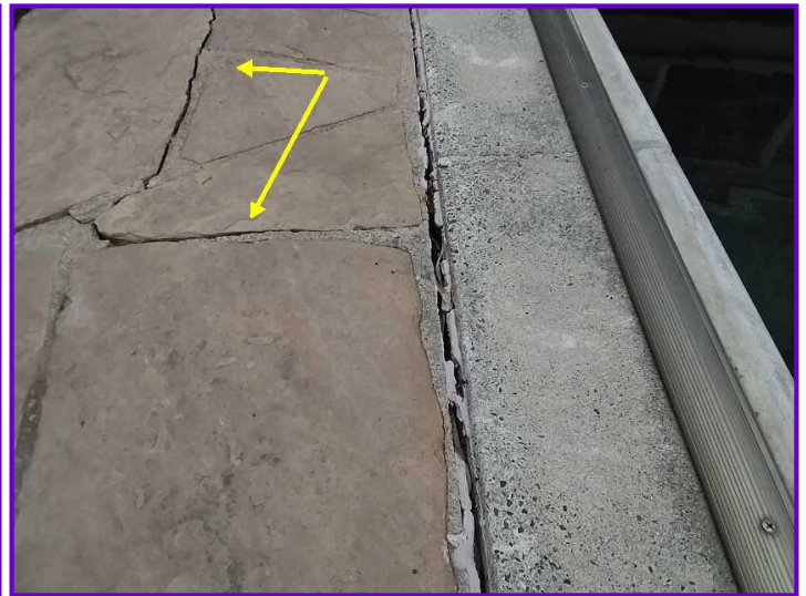
DEFERRED: The pool deck is cracked at multiple location.
