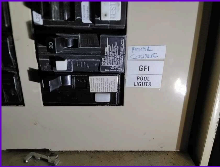
COMMENTS: The pool light circuit appears to GFCI protected as required for safety.
