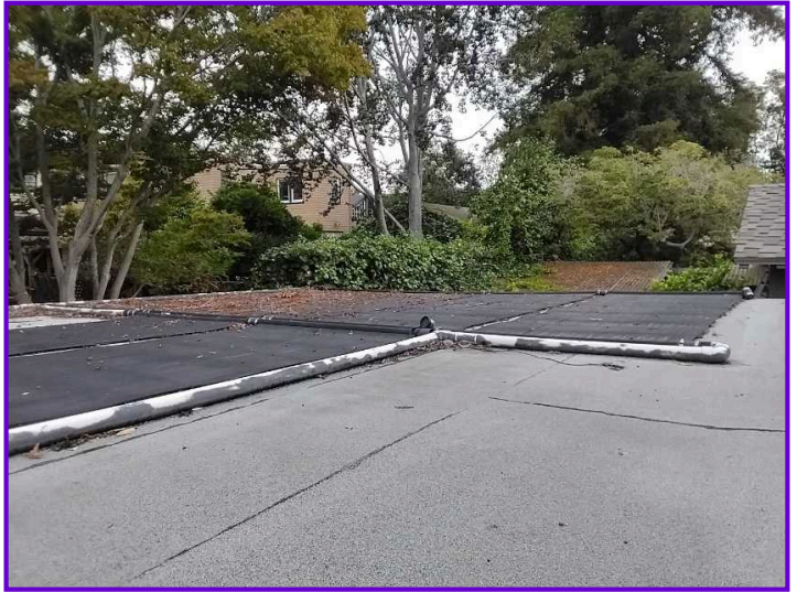
DEFERRED: The pool plumbing includes a hydronic solar panel water heating system located on the garage roof.
