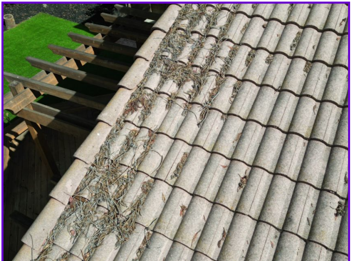
PREVENTIVE: Regular cleaning and maintenance of the roof are essential.
