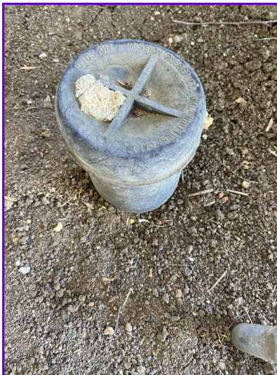
COMMENTS: The sewer lateral access and cover were observed to be in good condition at the time of inspection.
