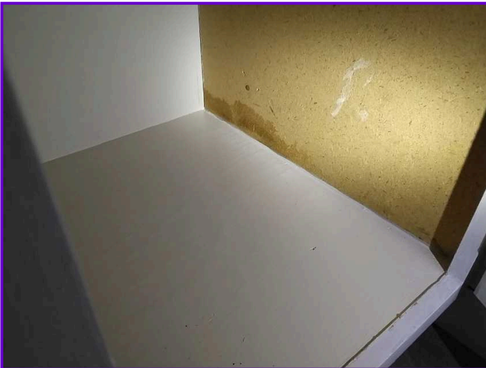
DEFERRED: Moisture stains were observed in the bathroom cabinet, likely caused by a previous leak under the sink.
