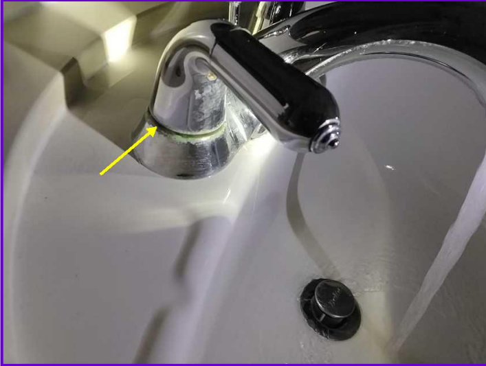
DEFICIENT: The faucet valves handle were leaking when in use.
