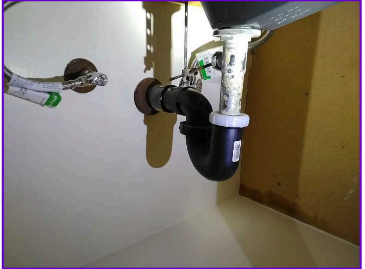
COMMENTS: The fixture drain and vent pipes within the property were functional.
