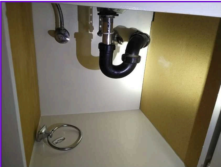
COMMENTS: The fixture drain and vent pipes within the property were functional.
