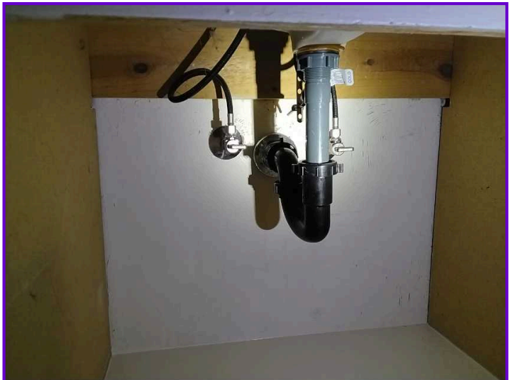
COMMENTS: The fixture drain and vent pipes within the property were functional.
