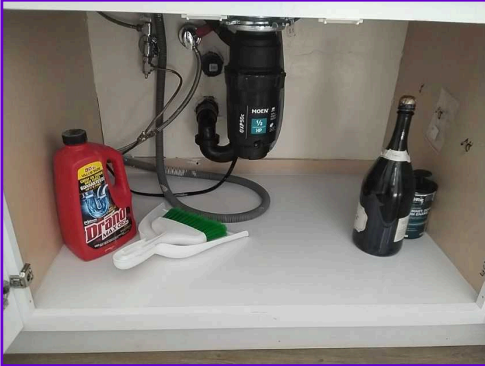
COMMENTS: The fixture drain and vent pipes within the property were functional.
