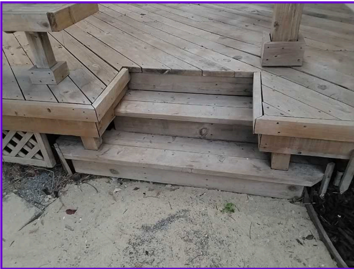
COMMENTS: The attached stairs and landing at the rear of the residence are in satisfactory condition.
