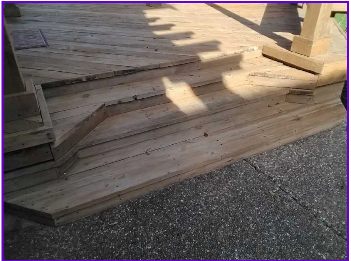
COMMENTS: The attached stairs at the rear of the residence are in satisfactory condition.
