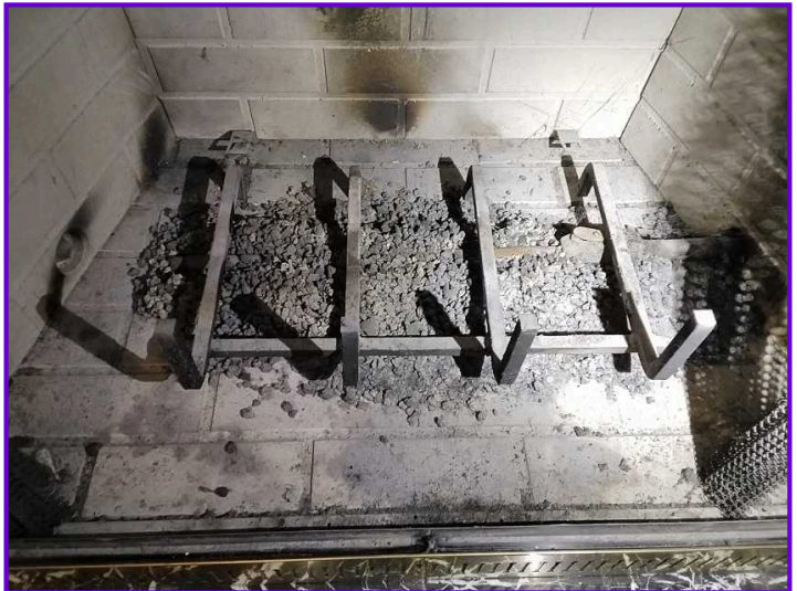
COMMENTS: The log grate appeared functional.
