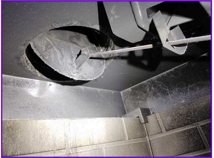
COMMENTS: The damper is functional.
