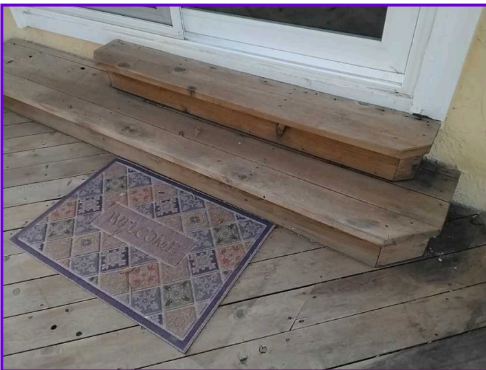
COMMENTS: The attached stairs at the rear of the residence are in satisfactory condition.
