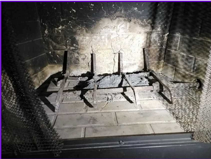
COMMENTS: The log grate appeared functional.
