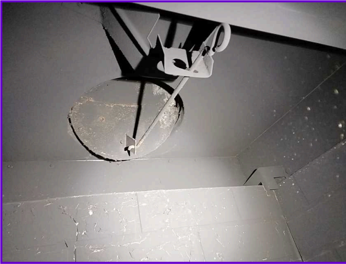
COMMENTS: The damper is functional.
