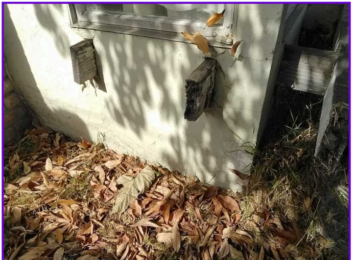
PREVENTIVE: A minimum 6 inches of clearance from the siding to the soil is needed at multiple locations around the residence.
