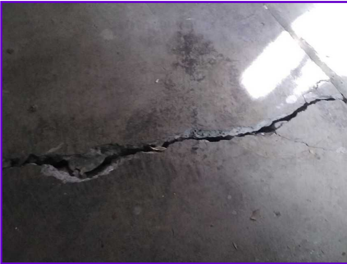
DEFERRED: There are significant separations in the garage concrete slab.
