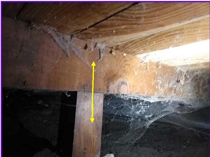
PREVENTIVE: Strengthening of the pier and post with metal ties or straps is recommended as a preventative measure.
