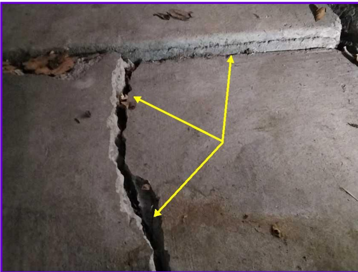
DEFERRED: There are significant separations in the garage concrete slab.
