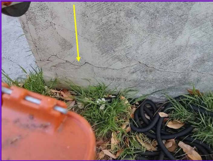
PREVENTIVE: There horizontal cracks in the stucco along the base of the walls.
