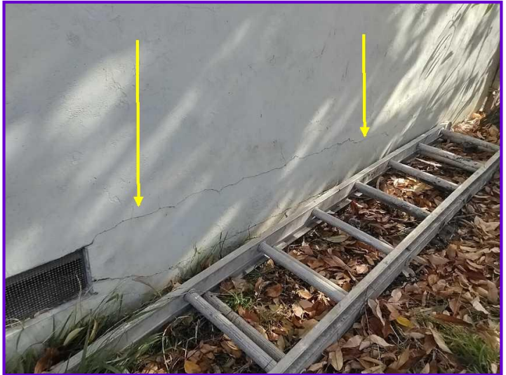
PREVENTIVE: There horizontal cracks in the stucco along the base of the walls.
