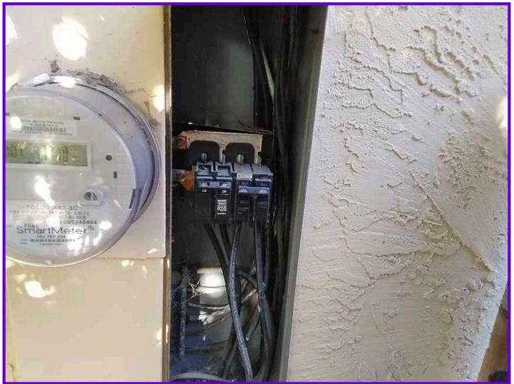
PREVENTIVE: The interior cover for the main electrical panel is missing.
