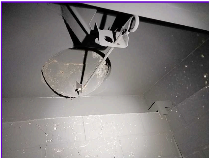
COMMENTS: The damper is functional.
