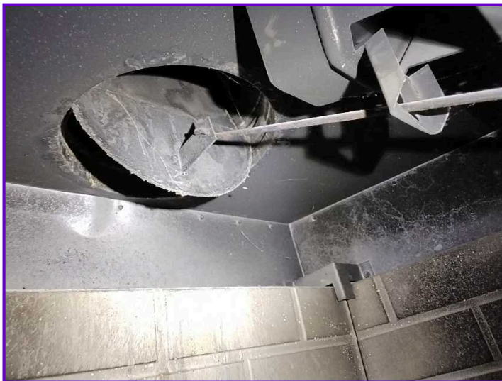
COMMENTS: The damper is functional.
